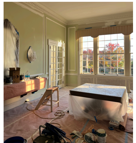
Repainted Dining Room after failed heating pipes damaged walls and ceiling
