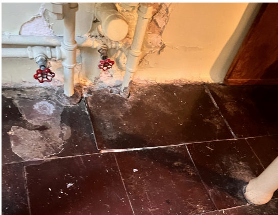
Leaking steam pipes in Kitchen wall creating havoc
