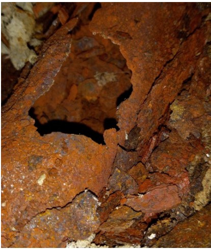
Crumbling, cracked, failing pipes in the Furnace Room
