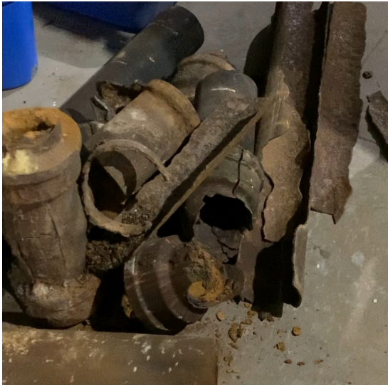
Excavated broken pipes in basement
